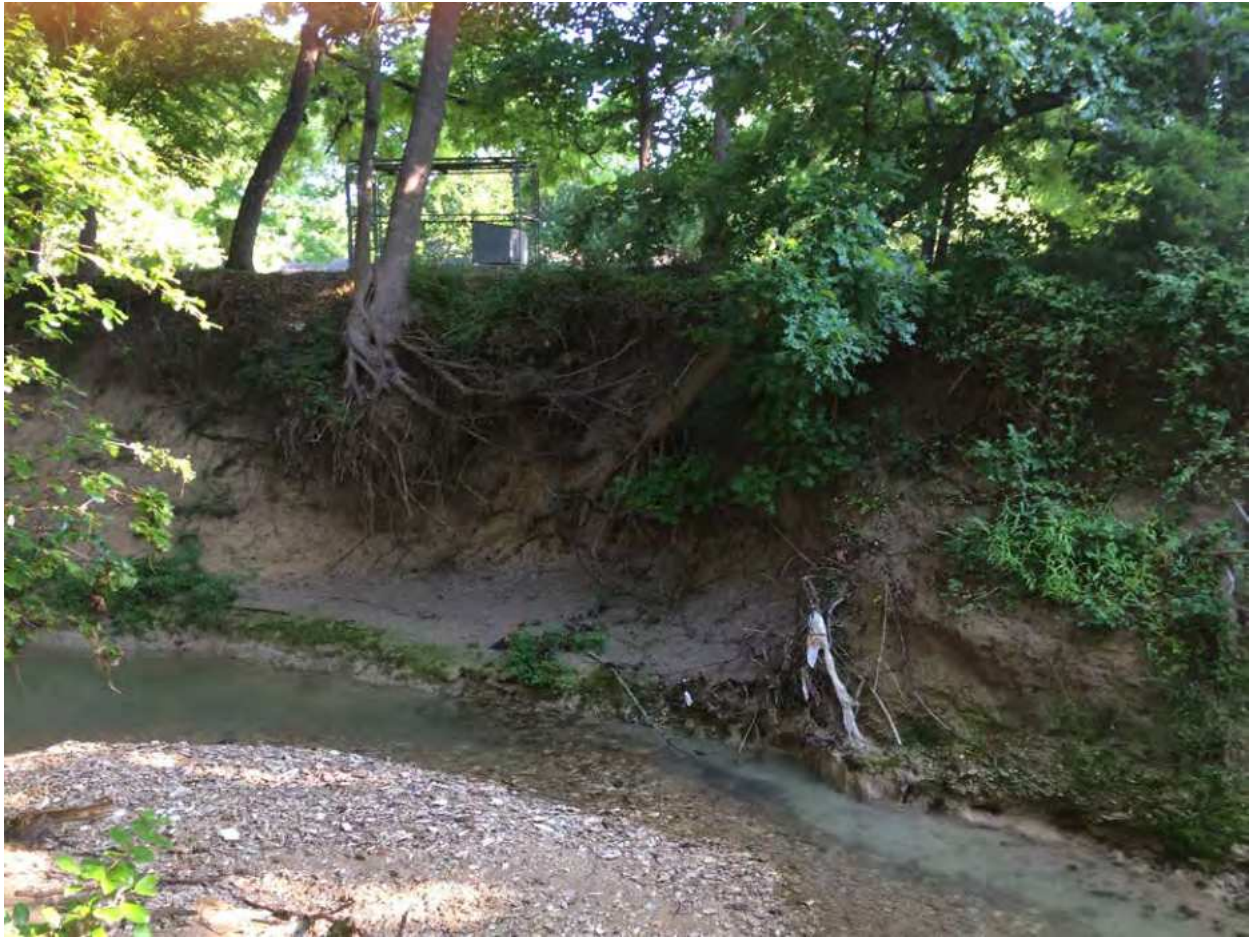
Severe erosion at stream outer bank
