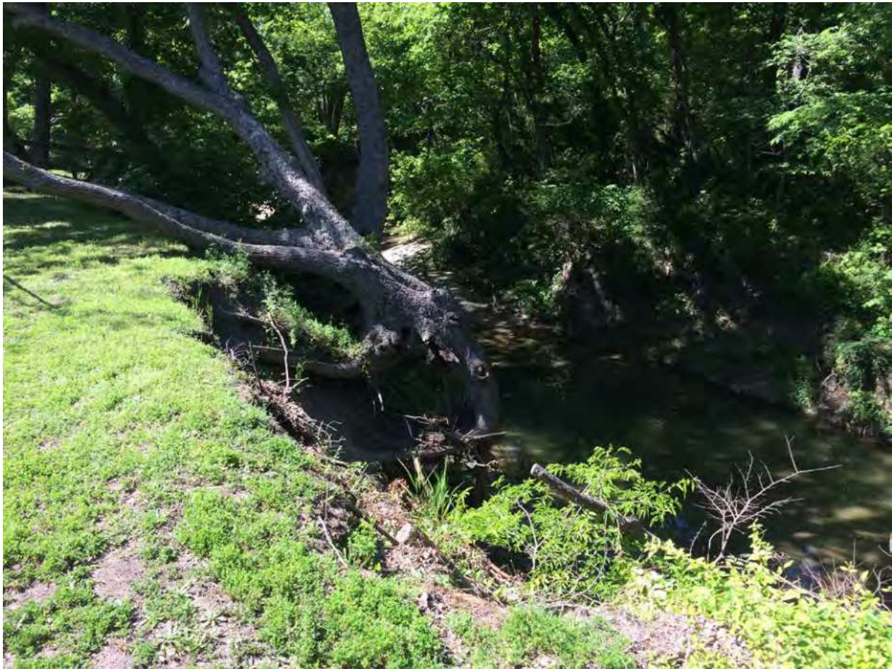
Severe bank erosion causing tree uprooting and loss of overbank
