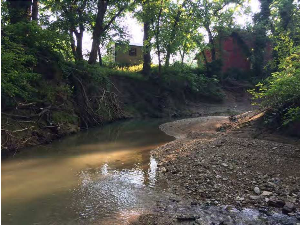
Bank erosion in the outer bend, and aggradation in the inner bend.
